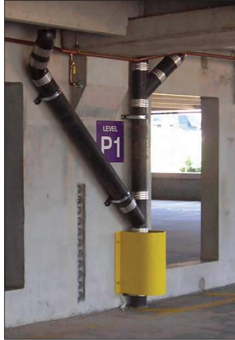
Figure 3-4 Drain Pipe Bumper Protection
