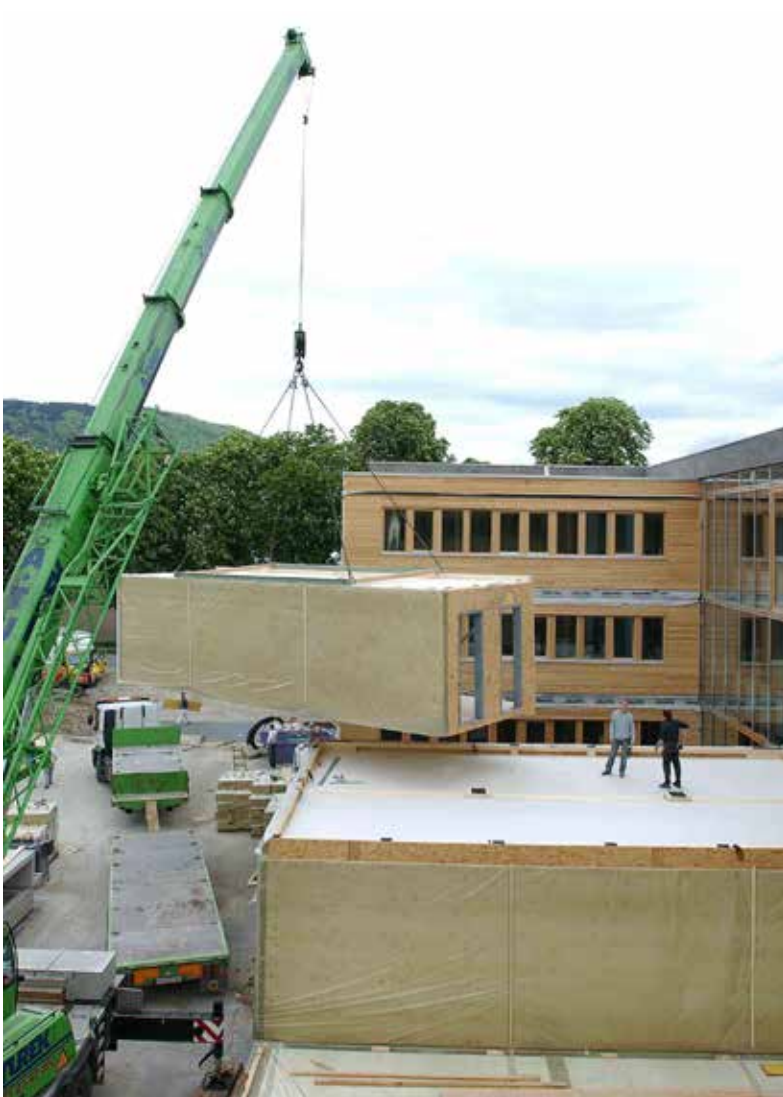
Figure 24 Impulsezentrum, Graz, Austria (courtesy of KLH)
