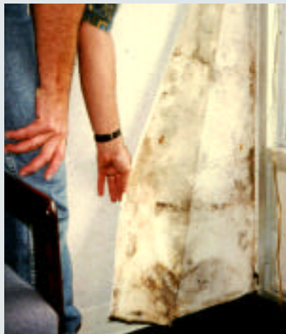
Mold growth behind vinyl wall covering.
