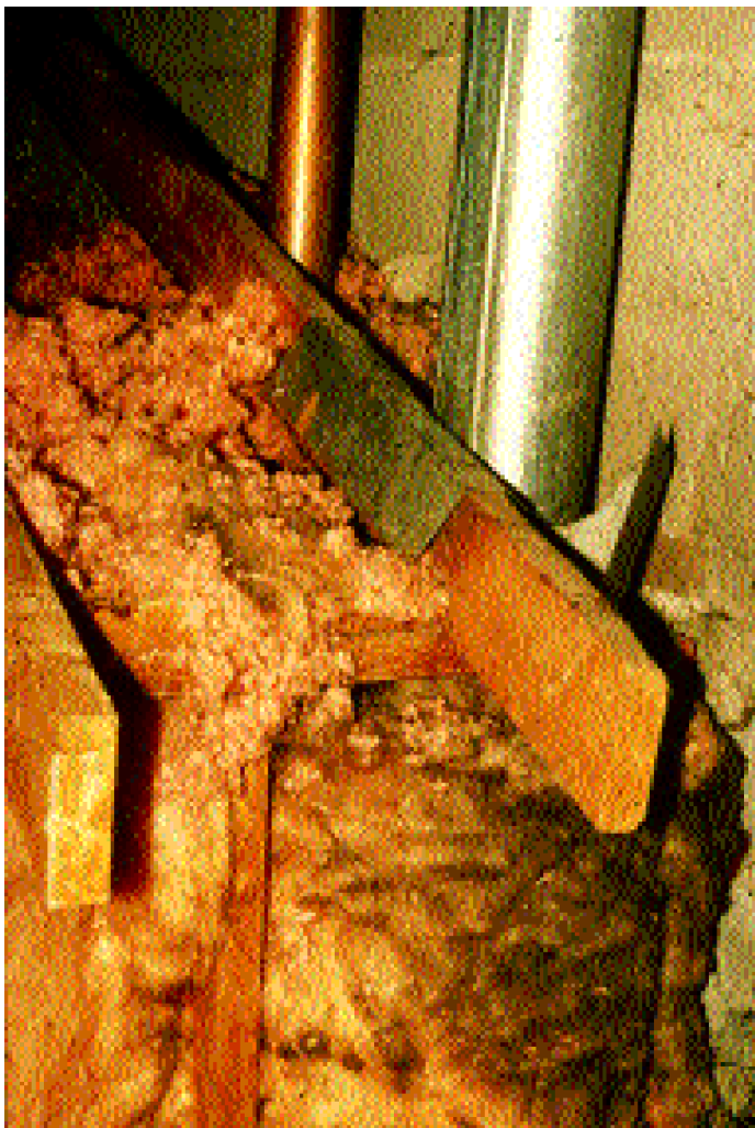
Fiberglass insulation is a filter, not an air-barrier. Note the dark markings (filtered dust) in the material.
