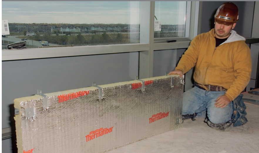
Impasse® hangers and locking washers are installed into Firespan® curtain wall insulation before inserting the insulation into the spandrel area.
