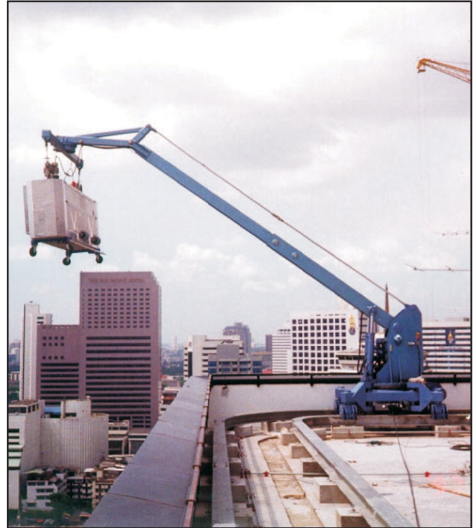
Roof car with traction hoists and wire winders on platform. Platform is 10'-0" (3 m) long.
