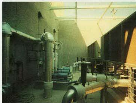
San Andreas Water Treatment Plant , San Francisco, California Engineer: Camp Dresser & McKee
