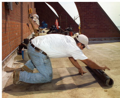
A roofing worker in the photo, top of the page, is seen cutting old roofing membrane into strips. Directly above, a worker rolls up the membrane prior to tack-welding the edges and placing it in the recycle container.
