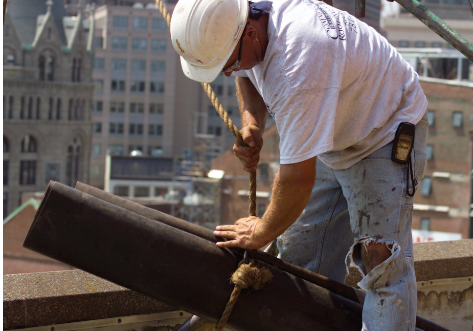
Rolls of old roofing membrane being readied for hoisting off the side of the building to the work area below.
