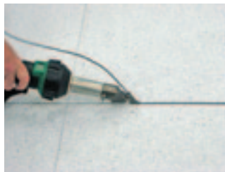
Welding bead is placed in the groove and fused by heat application.
