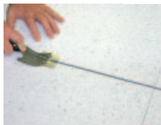
Welding bead is trimmed in two steps, with an initial trim using a trim plate.
