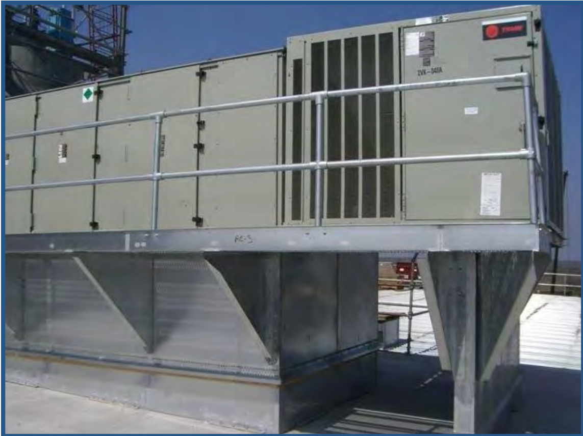
Full Perimeter Catwalk with Condenser Rail
