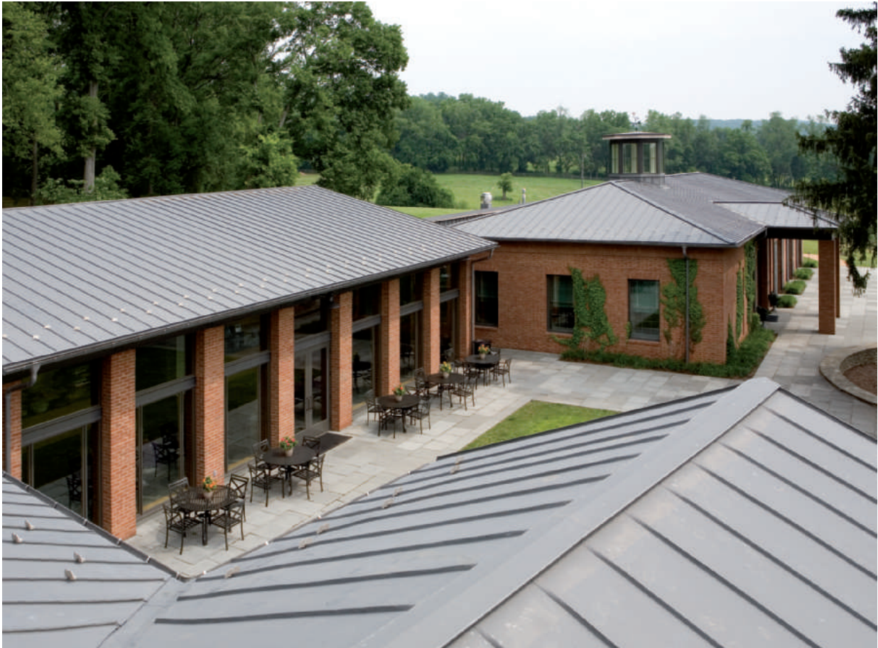
Standing seam (QUARTZ-ZINC ® ) James Madison's Montpelier Visitor Center (USA) Architect: Glave & Holmes Associates Installer: International Roofing
