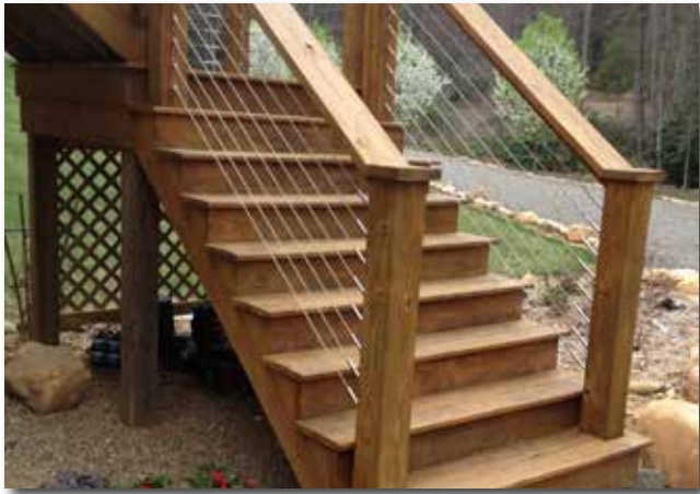
Private Home - Celso, NC Cable Fabricator: Charleston's Rigging & Marine Inc. Charleston, SC
