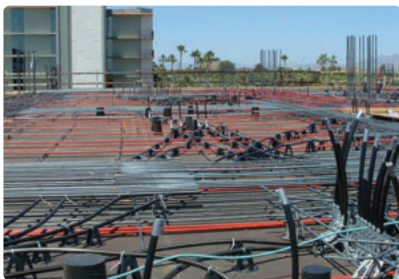
Tube-in-tube application for a potable water system embedded in the concrete pour
