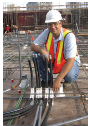
Uponor plumbing system in Lanikea, Honolulu
