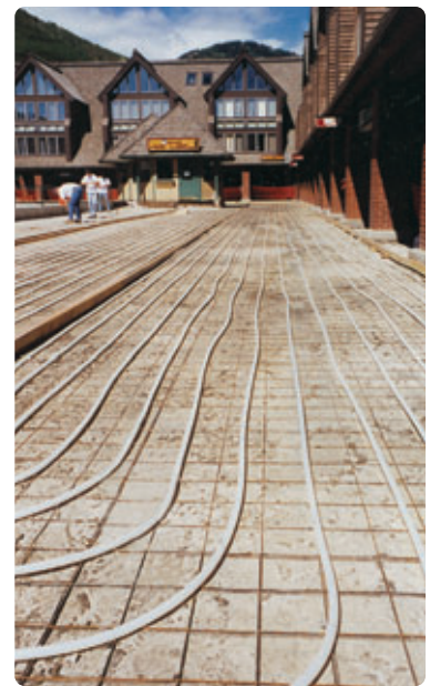
Installation photo from a ski resort in Park City, Utah
