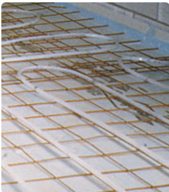
PEX tubing installed with mesh over insulation
