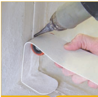
Fig 1: Waterproofing Details – Waterproofing Plus system which has built in extra protection on all critical details.
