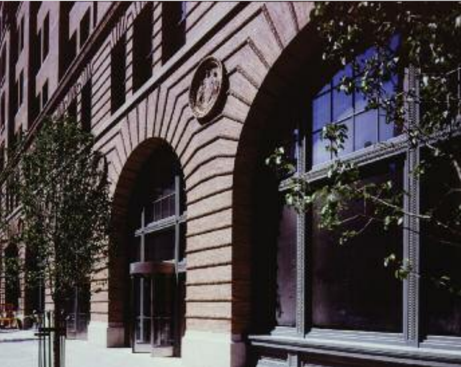
Baruch College New York, New York Site A building renovation 25th and 26th Street storefronts Baruch College – CUNY
