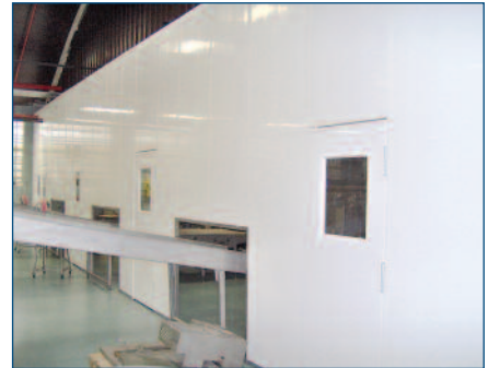
12 Foot High Wall with Double Swing Doors and Conveyors for Process Room
