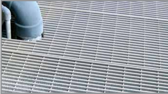
▲ WWTP - Youngstown, OH
