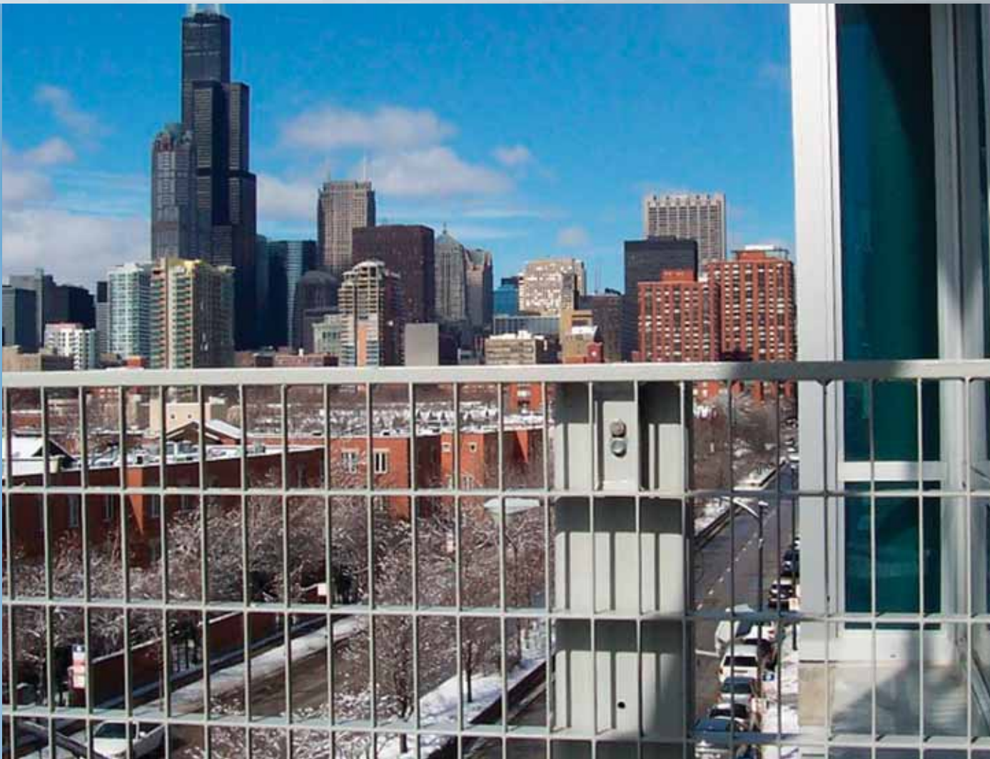
1401 S. State Street Balcony Handrail ▲ - Chicago, IL
