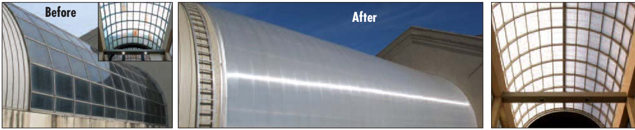
ID 13242 - Prime Osborne Convention Ctr., Jacksonville, FL Architect: Manousa Lewis & Dodson Architects, Tallahassee, FL CPI replaced an old failed leaking glass skylight with a Quadwall® system and retrofitted the existing structure. Skinning the structure with one continuous panel system from the sill to the apex eliminated any transverse connections.
