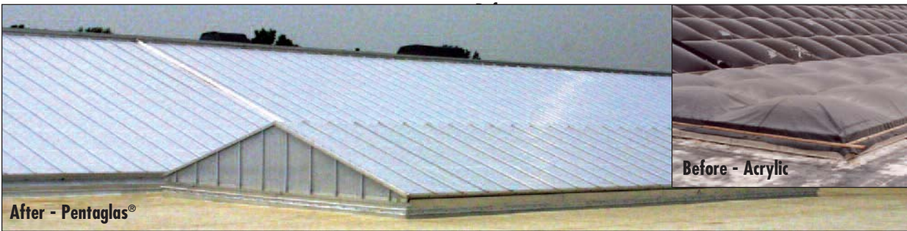
ID 9228 - Hazlewood East High School, St. Louis, MO CPI provided a solution to two clusters of leaking acrylic skylights by creating a heat-bent ridge skylight over one flat area of the skylight clusters and a single slope skin system over the other existing skylight clusters.
