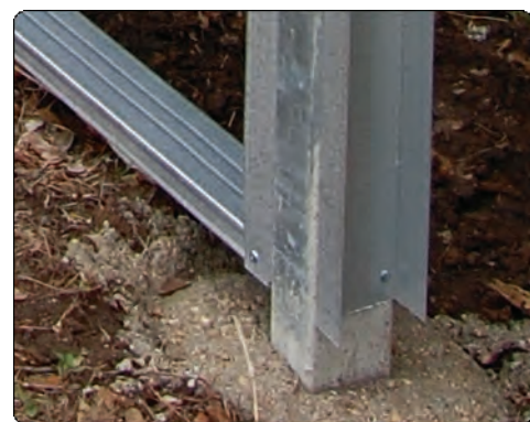
24 GA Track fastens vertically to 16 GA C-Channel Posts on both sides to receive 24 GA horizontal studs.
