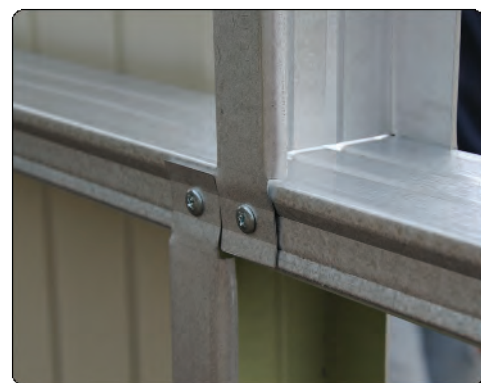
Detailed view of prefabricated vertical blocking members attached to horizontal metal studs.
