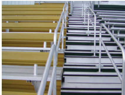
Handrails and Substeps
