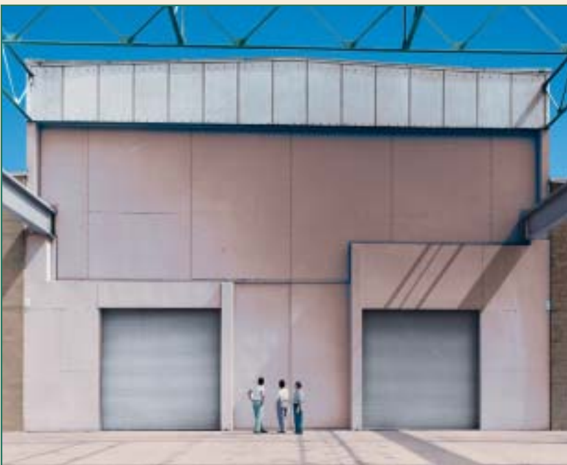
Note the asymmetrical profile of the Craneway Door Leaf accommodating the different heights of the partition walls.
