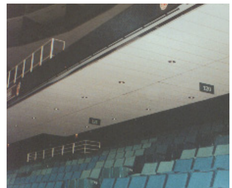
▲ Lay-in Ceiling Panels Miami Heat Arena, Miami, FL
