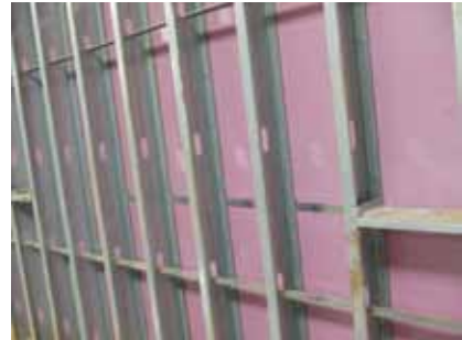
Figure 3 Combination of horizontal bracing through the steel stud knockout and a steel strap on the outer flange of the stud.
