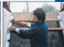
Cut wooden treads to required length and slide them into stringer slots.
