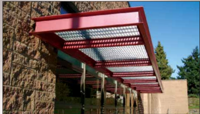
Aluminum Bar Grating works well for this school building sunscreen. Its appeal is durable, self-cleaning and allows adequate air movement.
