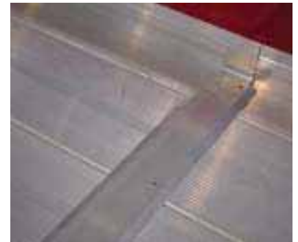
New beveled threshold splice cover
