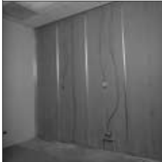
7. Flexible prewired electrical systems can also be used in ULTRAWALL partition systems. Photo illustrates one side of wall erected with T-studs prior to electrification.
