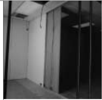
12. Outlets occurring in adjacent wall cavities can be handled by independent cables dropped from above ceiling...
