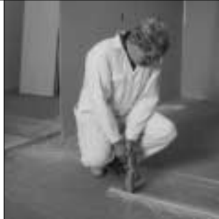
8. At door openings and freestanding wall terminations, anchor floor runner to subfloor.
