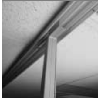
Method 3. Cut and bend strut runner to overlap strut legs and inner flanges of ceiling runner. Screw-attach strut to ceiling runner at corners.
