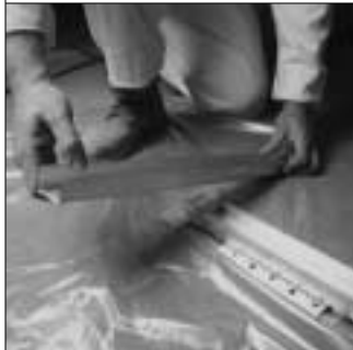
10. At intersections of floor runners with carpet grippers, cut and flatten legs of one runner to accommodate lapping of runners and positioning of wall panels.
