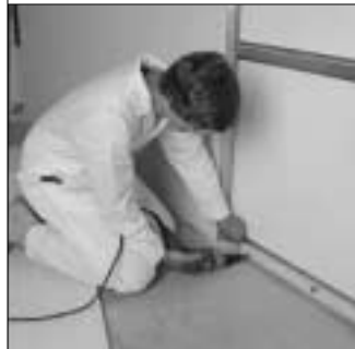
13. 1/4-in. wood strips are applied to face of existing wall to provide backing to panels at base. A 1-3/8"x7/8"x 24 ga. metal is required at the base for fire rated construction.
