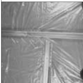
13. At floor runner intersections, floor runners can be secured directly to subfloor in lieu of screw-attaching them together. Note that intersecting runner is cut short to allow panel to pass through.
