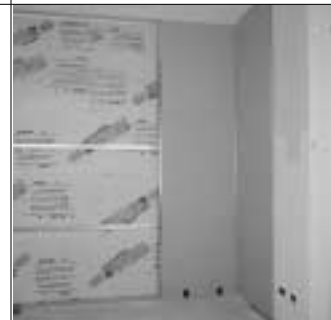
18. Supplemental horizontal members angle clipped to T-studs are required for partition rigidity.
