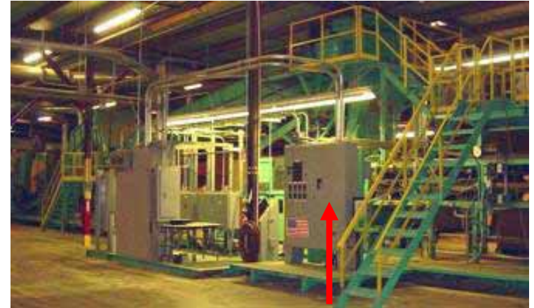
Compactor Control Center
