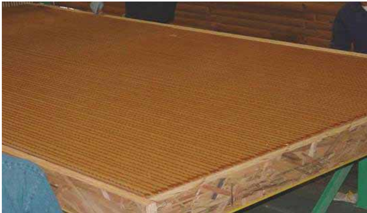
3rd Adhesive Layer Applied Between the CAF Core and the Top OSB Layer
