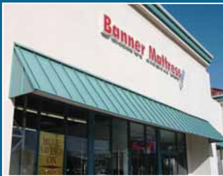
Pic. 07 | metal awnings
