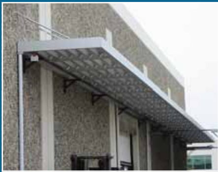
Pic. 03 | metal awnings
