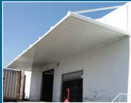
Pic. 08 | metal awnings
