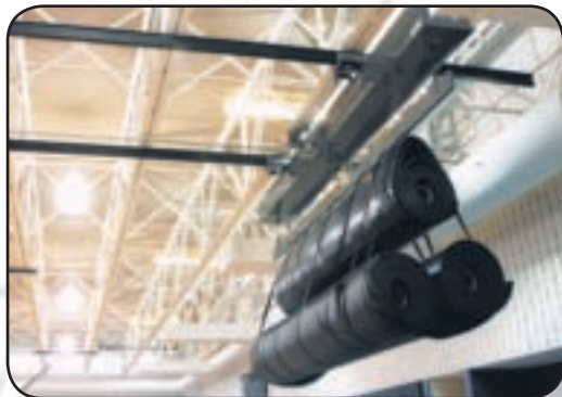
Sectional Mat Lifter with Sideways Traveling Kit, Hartland (MI) High School. Architect: Kingscott Associates, Inc. Photography: Wayne Williams, Indianapolis, IN.
