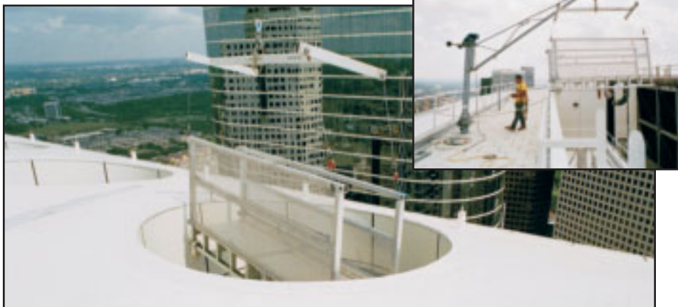
A section of a window cleaning platform is being lifted from a 40th floor roof storage area using a motor operated, demountable Pro-Bel winch-hoist. It is then swung across a promenade surface (inset photo) and then through a 10'-0" (3 m) diameter hole in a roof overhang for assembly on a lower roof. Enron Building 2, Houston Texas.
