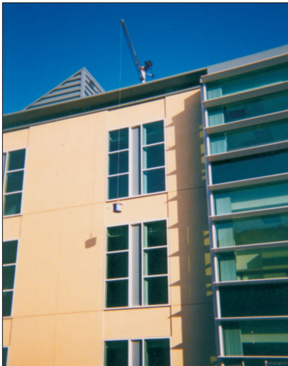
Winch-hoist being used to lift material onto roof. Travis County Criminal Justice Center, Austin Texas.
