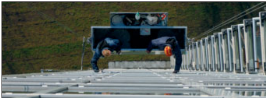
This birds-eye view of a permanent powered platform shows platform stabilizer ties secured to a horizontal cable attached to the building approximately every three floors.
