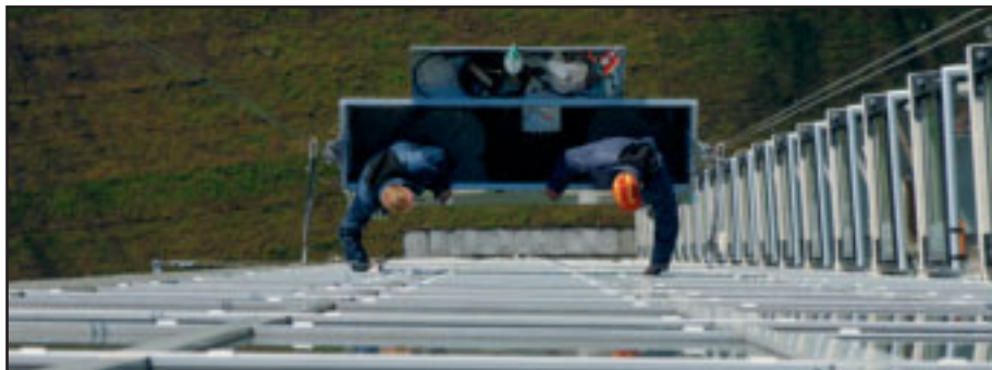
This birds-eye view of a permanent powered platform shows platform stabilizer ties secured to a horizontal cable attached to the building approximately every three floors.
