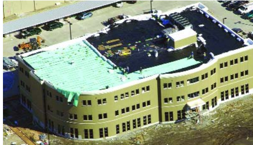
16,000 sq. ft. of EnkaRetain & Drain is being installed on the 251 Medical Center Blvd. project. Photo courtesy of Jacob White Construction.
