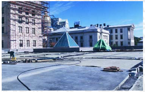
Preparation for the Enkadrain layer at the New Jersey State House roof garden project.
