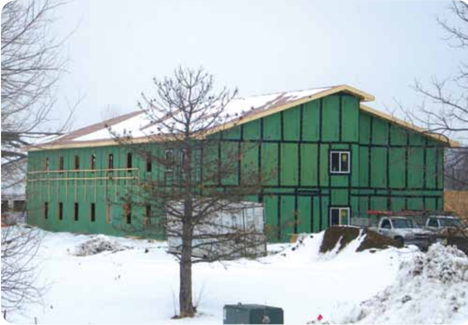
Trinity Village Papillion, NE Architect: Schemmer & Associates Owner: Immanuel Communities GC: The Weitz Company
