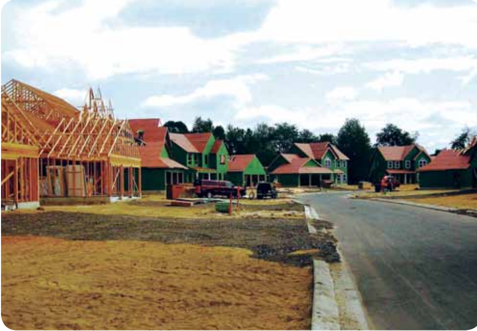
McGuire/Fort Dix Military Family Housing Fort Dix, NJ Architect: Woolpert, Inc. Developer: United Communities
