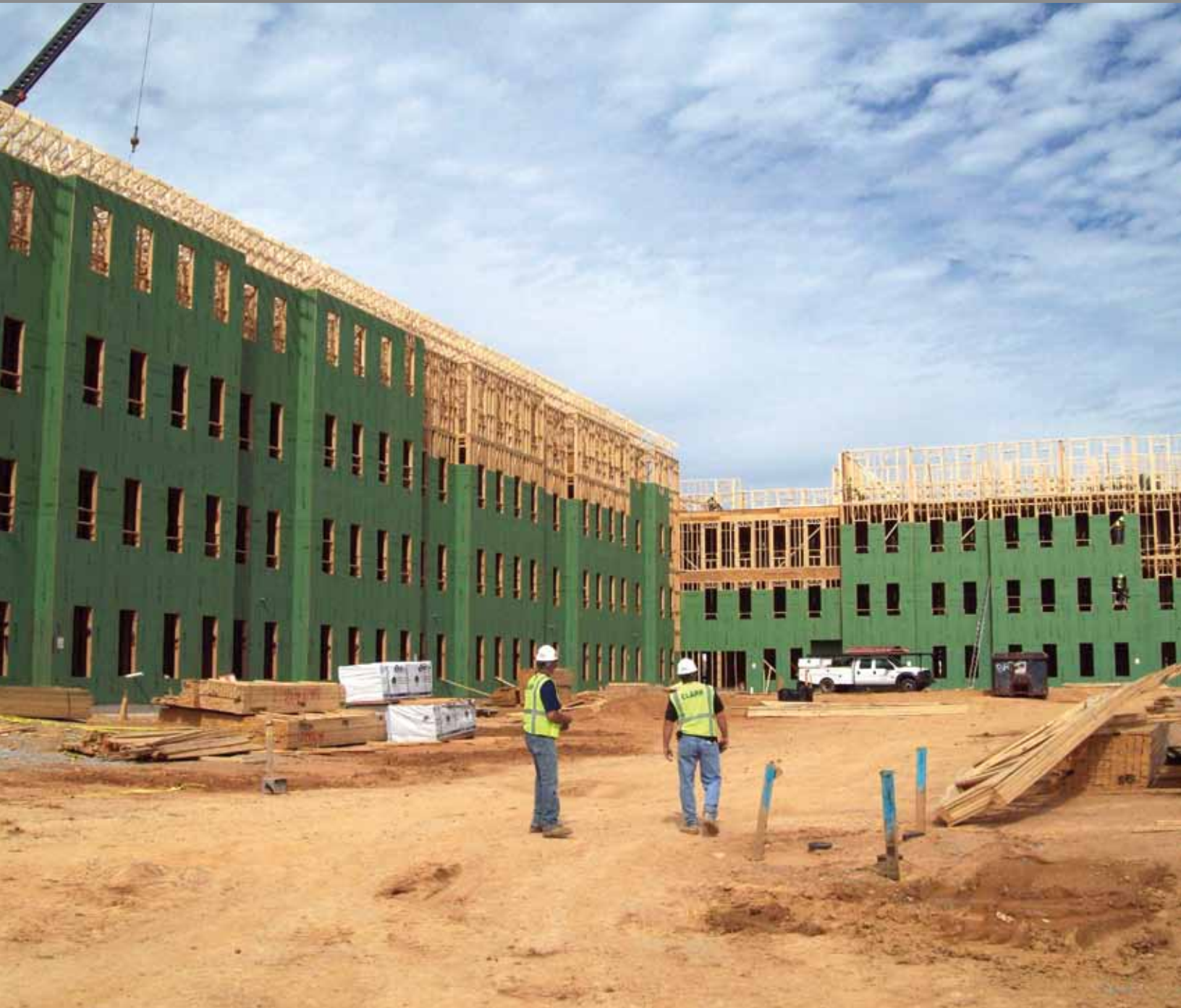
Fort Belvoir Warrior In Transition Housing Alexandria, VA GC: Clark Builders Group
