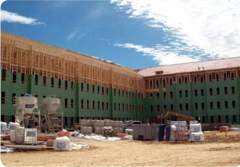
Fort Belvoir Warrior In Transition Housing Alexandria, VA GC: Clark Builders Group
