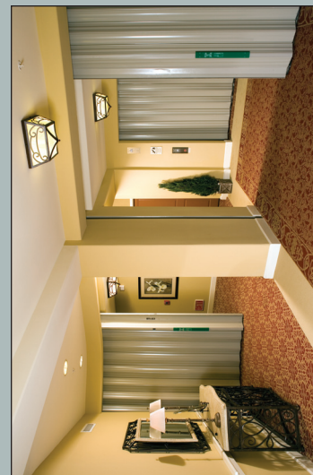
Now you see the fire-doors ...
